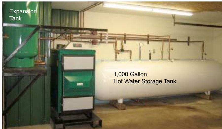
EKO 60 with 1,000 gallons of pressurized hot water storage and expansion tank.
