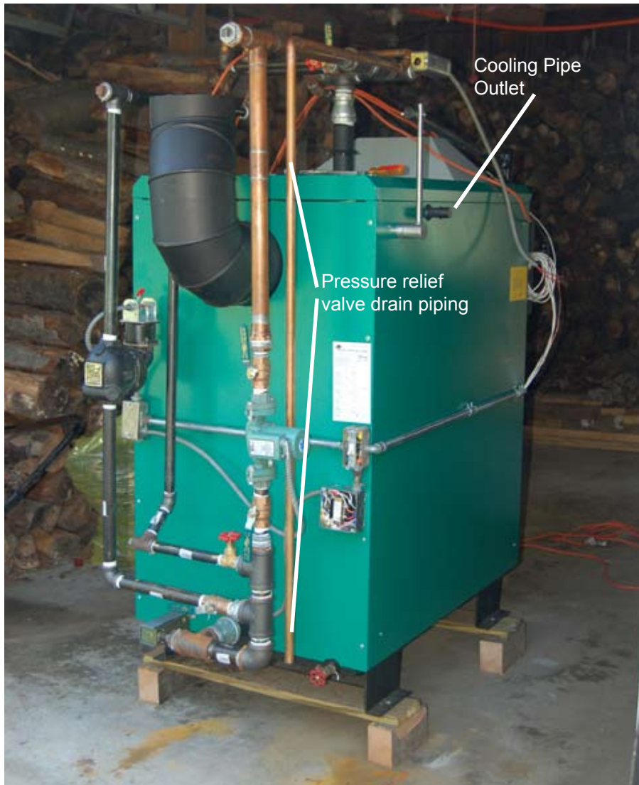
Photograph showing one of the cooling pipe outlets and the pressure relief valve piped to within 6 inches of the floor with rigid copper pipe.
