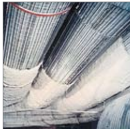
Protection incendie Fire protection
